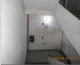
Photo of fire safety equipment Evacuation sign and emergency light at stair.jpg
