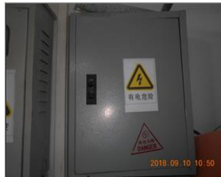
Photo of the inside of the main production hall Electrical box.jpg
