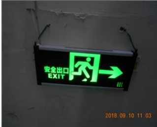
Photo of fire safety equipment Evacuation sign.jpg
